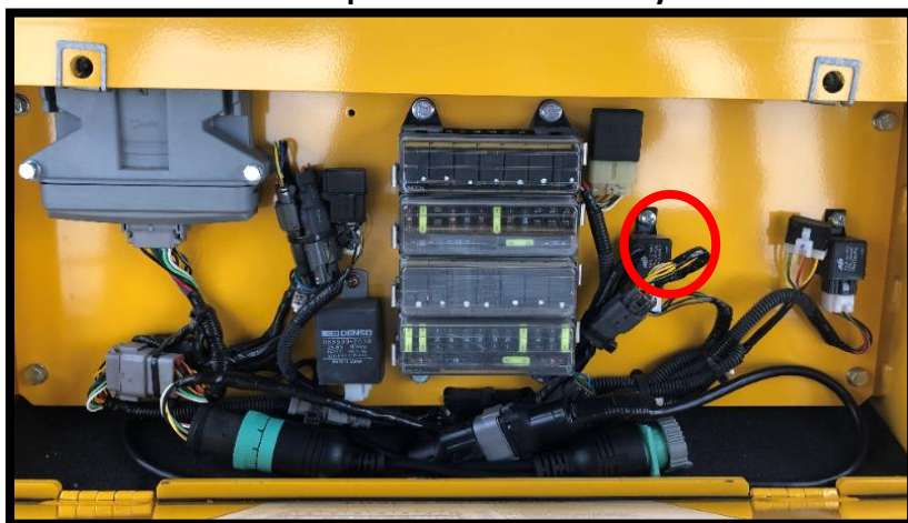
Pump Neutral Relay
